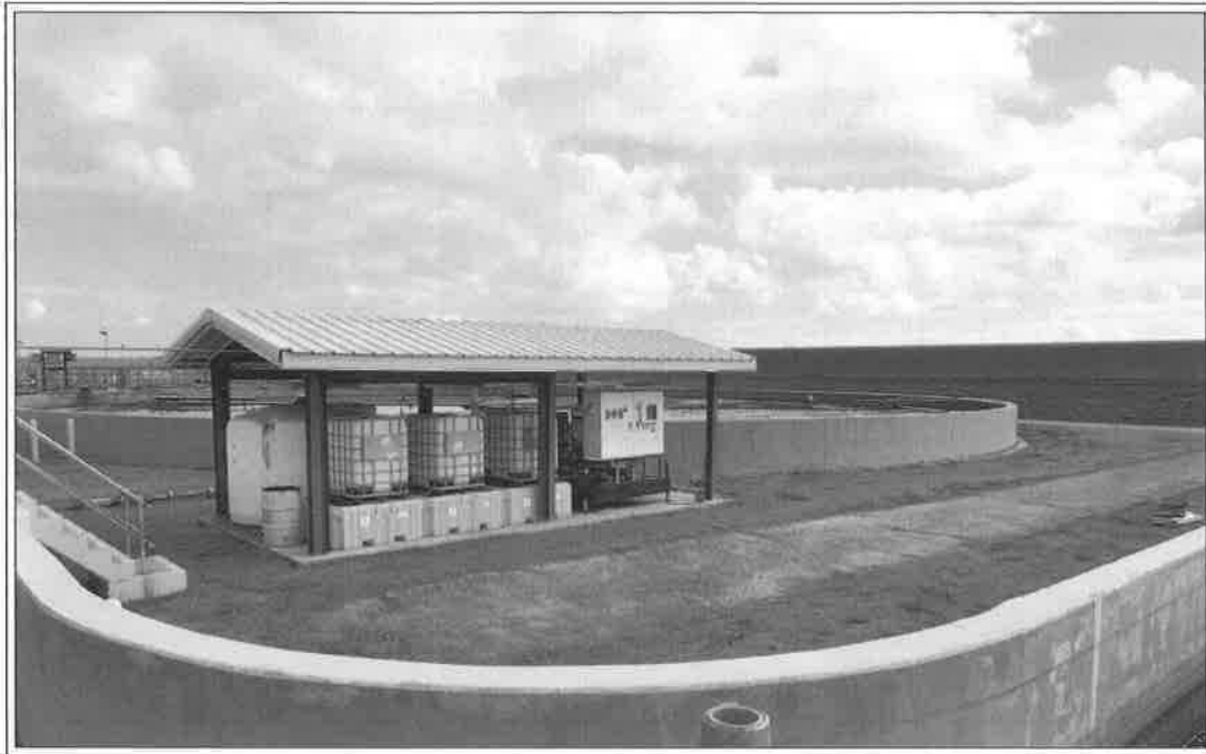
The ferrator system at the East Bank Sewage Treatment Plant is designed to fully disinfect the effluent prior to discharge to the wetlands, with no residual effects or by-products. This new technology is being used in a pilot trial with the wetlands. In the foreground is the current effluent channel where all of the water that is currently treated is disinfected prior to discharge to the Mississippi River. Behind the Ferrator is a Final Clarifier that will be the source of water used in the first phase of the Wetlands Assimilation project, a partnership with Orleans and St. Bernard Parishes.
