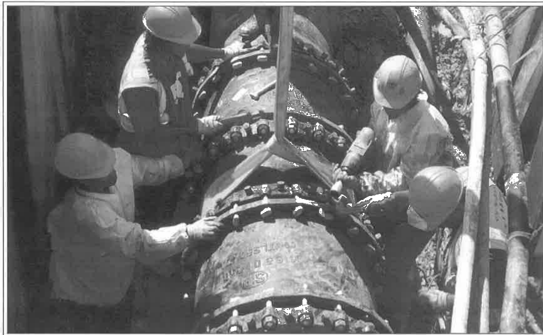
The City's aging infrastructure, soft soils, Katrina damage and the high number of tree roots result in numerous breaks in underground water, sewerage and drainage pipes and mains. And, even though the Sewerage and Water Board has crews on duty 24 hours a day to repair thousands of broken pipes, the number of new breaks continue to rise. A good example, shown here, is the repair of a break in a major 30-inch water main in the Carrollton area which also supplies water to other parts of the City. Complicating the repair of the 80-year-old pipe was the difficulty identifying other utility lines in the area and having them shut down. Because of the age and design of the old pipe, the Board's own Machine Shop of the Facilities Maintenance Department made sleeves and fittings to match with the old main. Their work shortened the repair time and saved money for customers.
